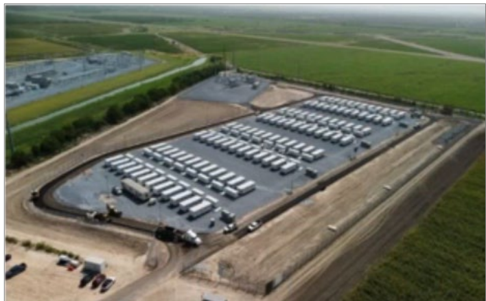
Eolian's 350 MW/1,400 MWh BESS system in Texas.
